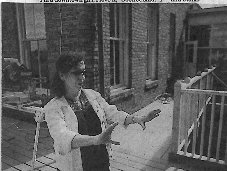
Karen Bruker describes where she wants the grill to go at their soon-to-be-completed home above her husband's office.
